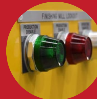
AC AND DC DRIVE UPGRADES
