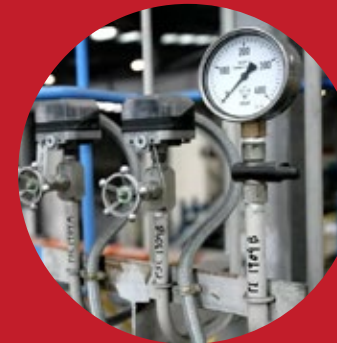
ROLLING MILL CONTROL
